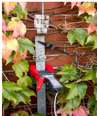
Current clamp to measure current at an individual ground point
