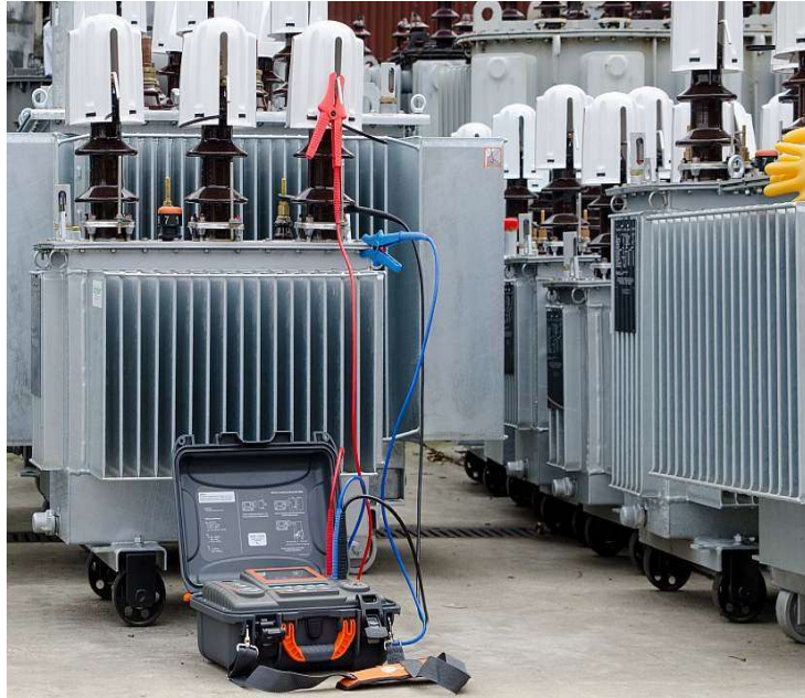
Sonel insulation test set operating in field conditions.
